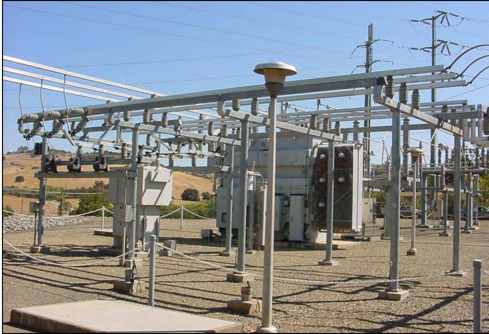
Figure 5. Typical Substation Equipment
