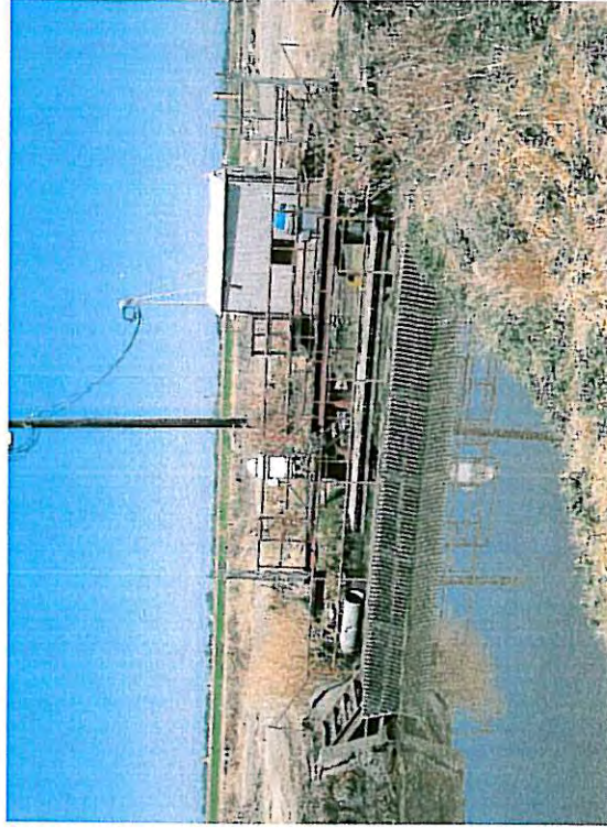
Pump station at E/W - N/S intersection approximately 3,000 feet south of Pacific-Riego Road intersection, view to northeast.
