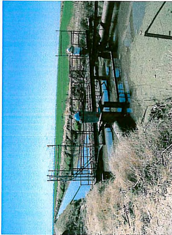
Pump station at E/W - N/S intersection approximately 3,000 feet south of Pacific-Riego Road intersection, view to northwest.
