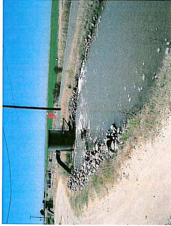
Pumps at East/West drainage, south of Riego Road, view to west.
