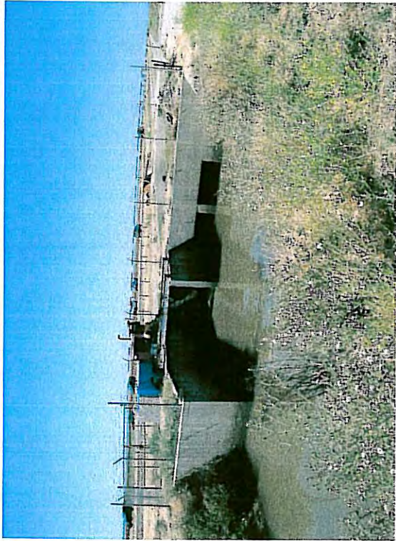
Drainage station east of Hwy 99, approximately 3,000 feet south of Riego Road, view to north.
