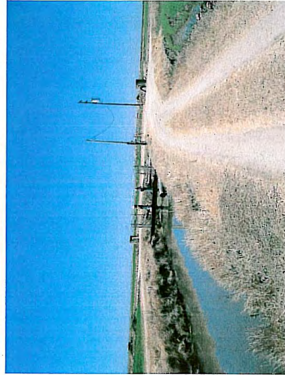
Pumps at North/South drainage, south of Riego Road, view to north.
