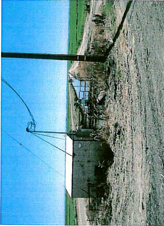
Pump station at E/W - N/S intersection approximately 3,000 feet south of Pacific-Riego Road intersection, view to west.
